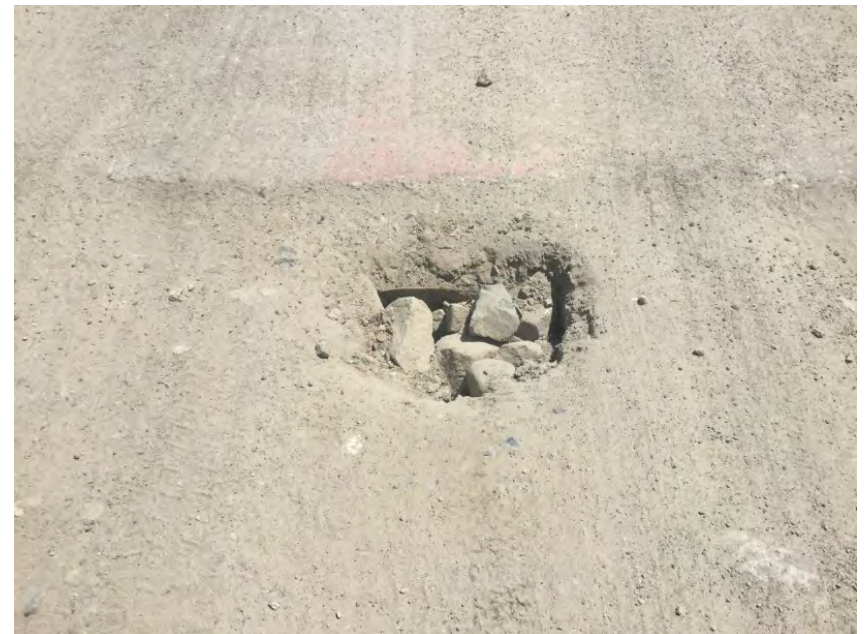
Hole at right approach
