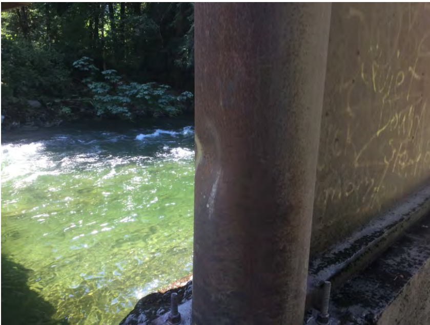
Damage to upstream pier column
